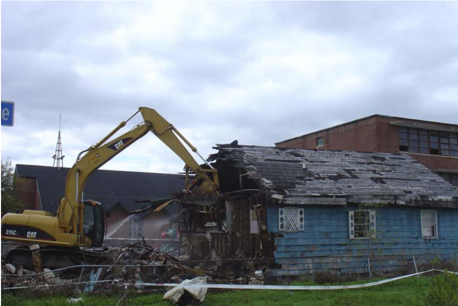
Figure 7. Unauthorized demolition in historic district, 2008.
